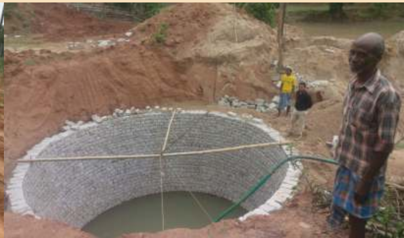
First installation of Lift irrigation under JOHAR project in Palkot block of Gumla District.
